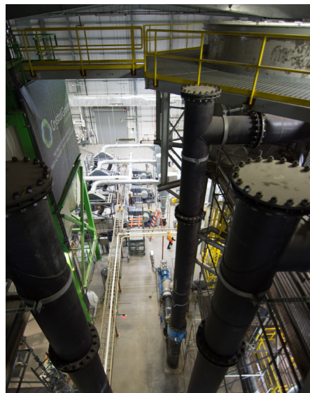
The MWRD's nutrient recovery facility with its three mega-sized reactors can recover more than 85 percent of the phosphorus and up to 15 percent of the nitrogen from the water cleaned by the plant.
