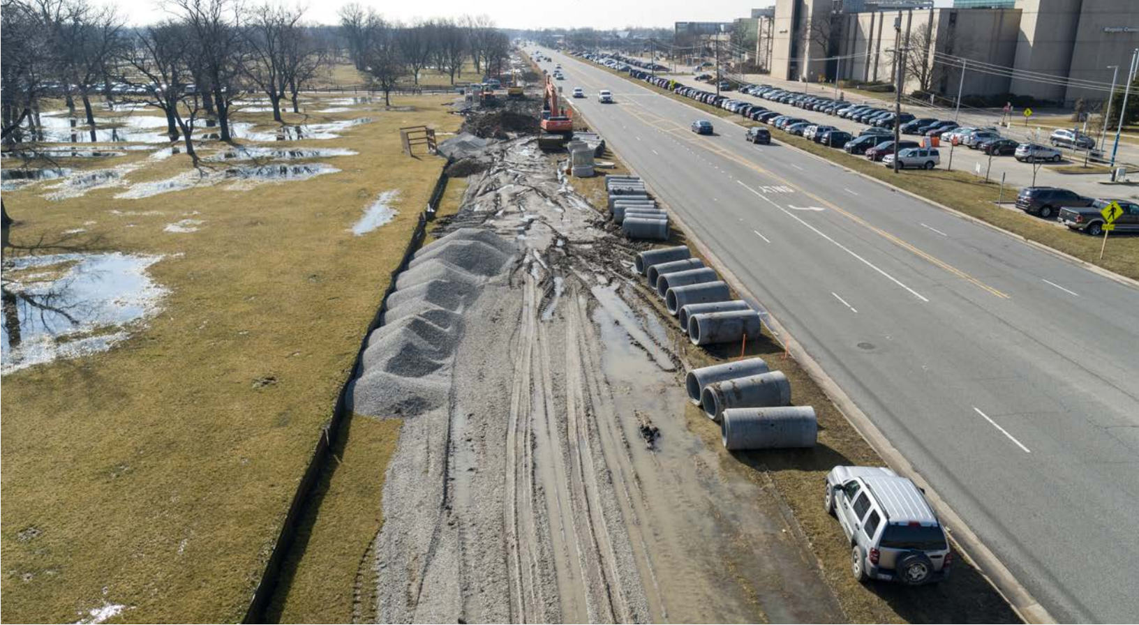
A view to the south shows excavation and placement of pipe during construction along 1st Avenue near Miller Meadow Nature Preserve in Forest Park.
