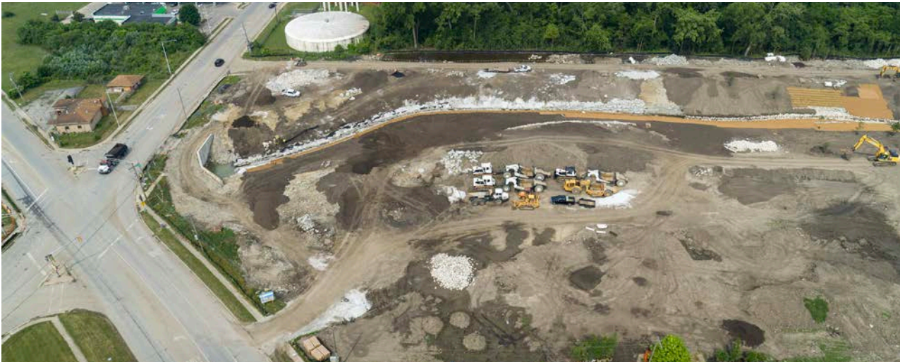
Excavation and construction at the Phase 1 area for the Robbins Heritage Park and Midlothian Creek Restoration Project.
