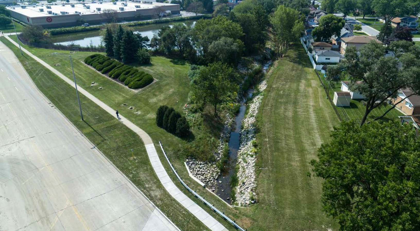
This ditch stabilization project provides additional storm and flood protection for more than 80 homes and structures throughout Crestwood.
