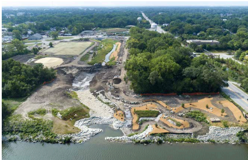
A southward view of construction for the MWRD's stormwater project in Robbins on the edge of the Cal-Sag Channel.
