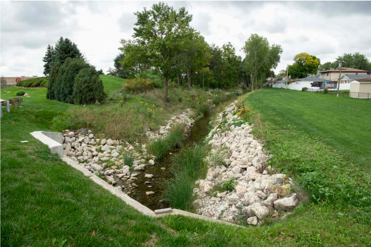
A view looking south from the new culvert under Cal-Sag Road in Crestwood, showing the improved Crestwood Drainage Ditch.
