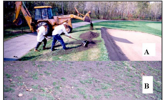
Photograph 4. Use of Bulldozer for Heavier Application of Biosolids to Roughs. (A) Before biosolids Application. (B) After biosolids Application.
