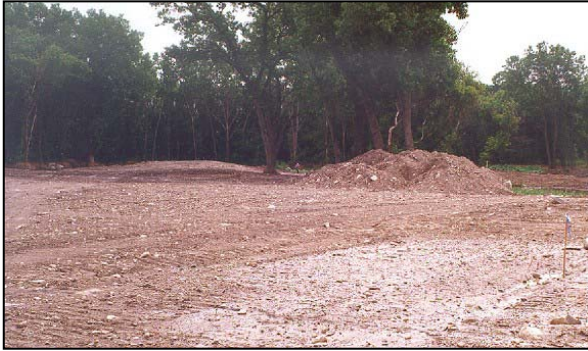
Photograph 1. A typical Fairway at the beginning of project. Note that stones and pebbles are clearly visible.
