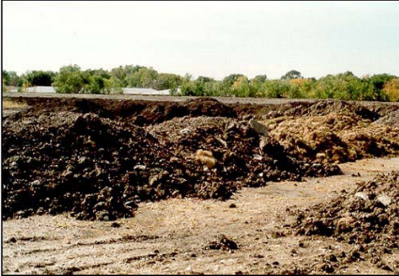
Photograph 1. Various types of fill materials stockpiled on the site
