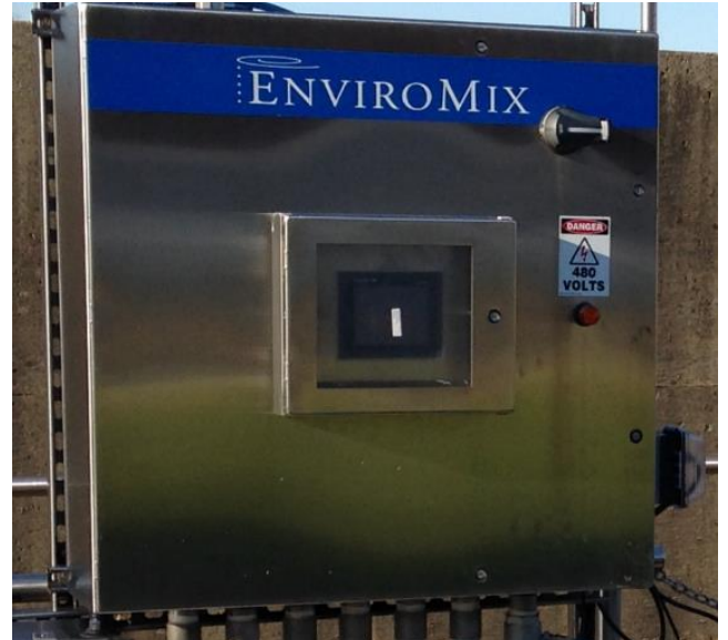
Valve Control Panel (VCP)
