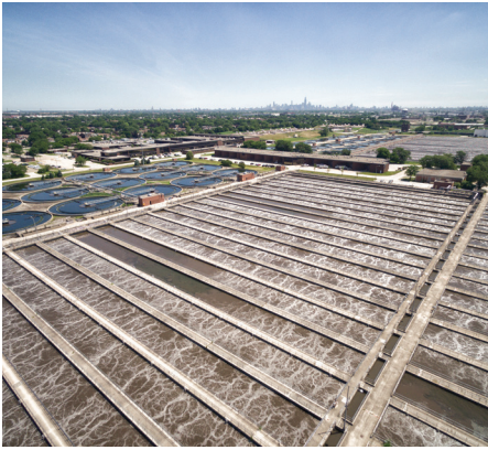
A biological process in 36 acres of aeration tanks removes suspended and dissolved solids from the wastewater.
